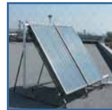
USKV-1 heater at Astrakhan-2 station of Privolzhskaya Railway
